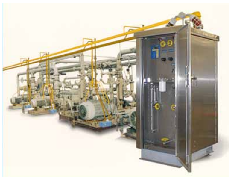
Figure 2 | Typical Enclosed Misting System (Courtesy of Colfax Corp.)
