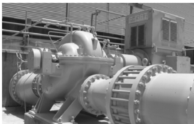
Figure 3 | Open System Pump Cooling Tower [Courtesy of Heinz P. Bloch, P.E. — Process Machinery Consulting]
